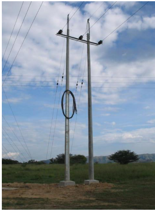
Torre Electrica A
